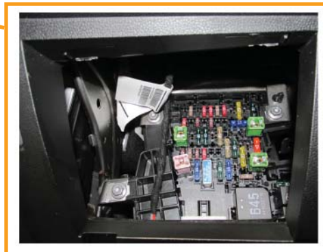
Relay and Fuse Holder SC at the Bottom Left of the Instrument Panel
